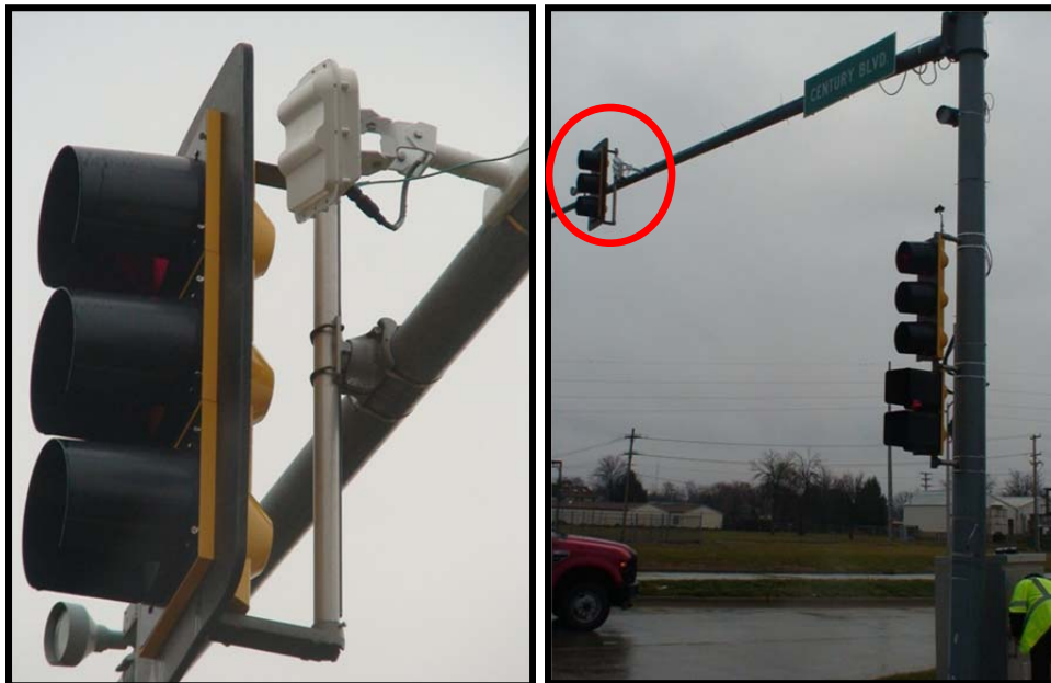
(b) Wavetronix Advance facing eastbound traffic and directed toward advance zones.
